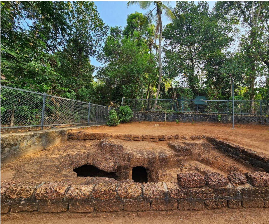
Image 7: Views of the monument showing loose laterite walls
